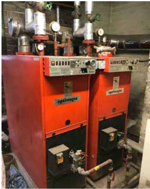
Two of the boilers for the church in the cellar of the house.
