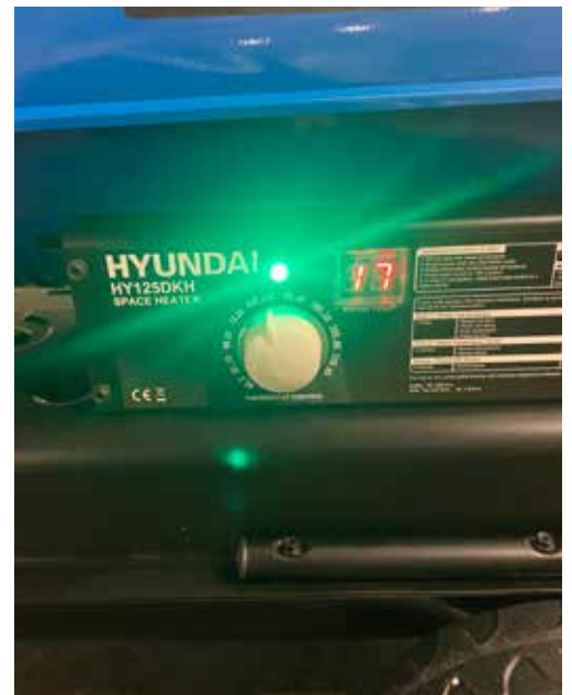
Picture taken on the 24 th December, showing the temperature in church, reached for the first time we used these heaters.
