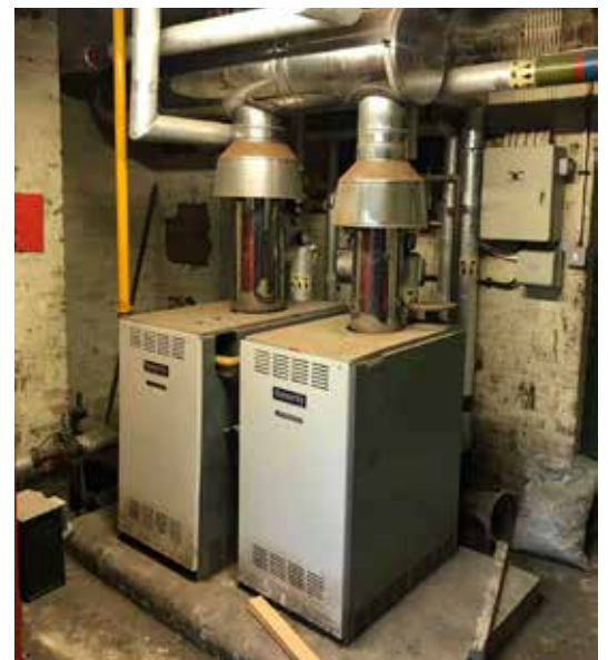
Opposite them, the other two boilers in the cellar. All boilers are over 40 years old, and have reached the end of their life.
